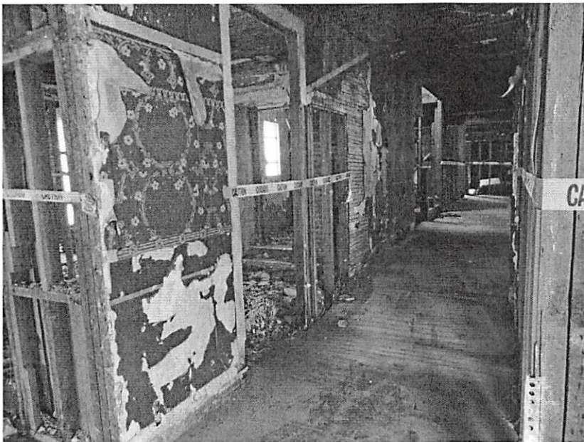
Figure 10: View of second-floor corridor of the Palace Hotel with partially removed plasterwork and non-contributing wallpaper
