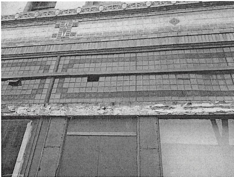
Figure 4: Detail view of prismatic glass transom at the exterior of the Palace Hotel
