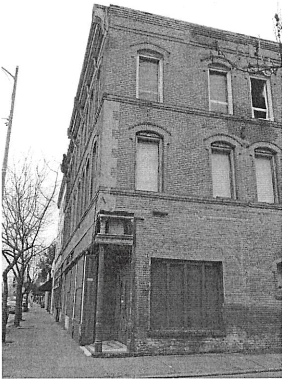
Figure 3: Exterior corner of the Palace Hotel with historic cast-iron column at the ground floor
